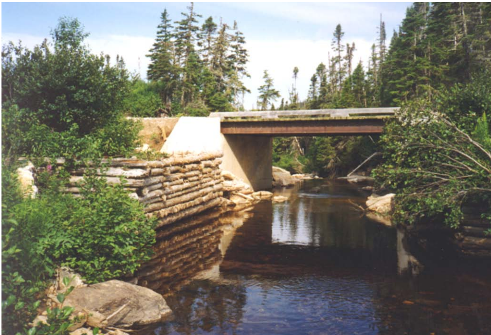
Figure 6-3. An example of old (log) and new (concrete) construction techniques for watercourse crossings.
