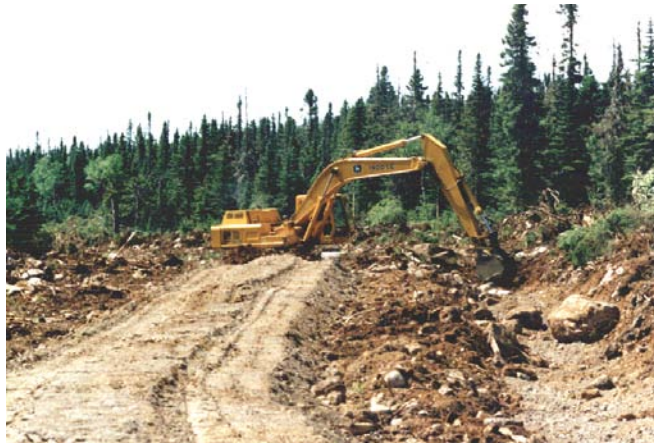
Figure 6-2. All forest access roads are constructed using excavators, which minimize site disturbance .
